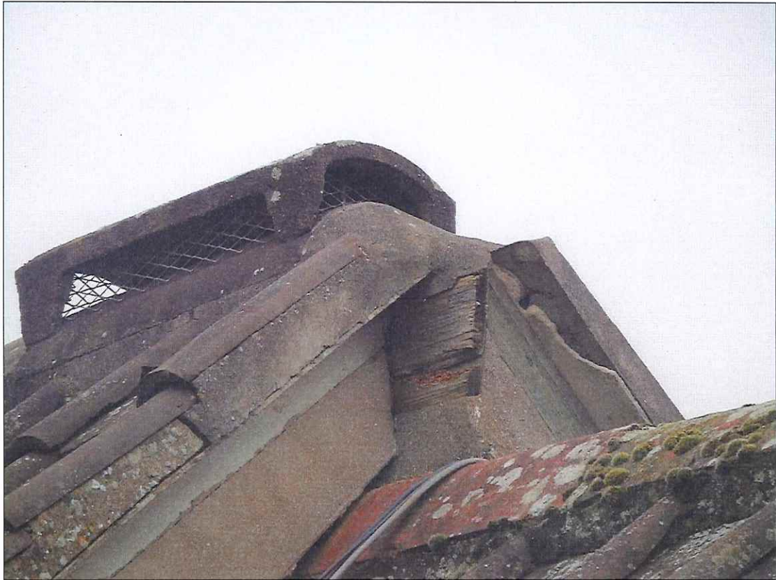
Rot to exposed ridge timber
