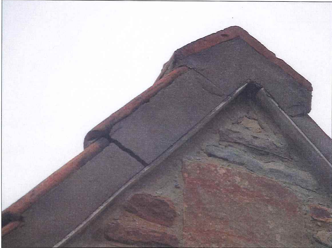
Cracked cement verge – rear gable
