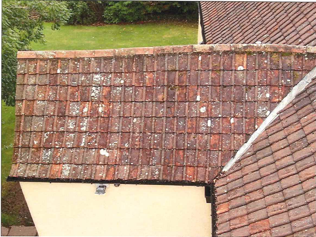
Front gable roof – slightly uneven ridge
